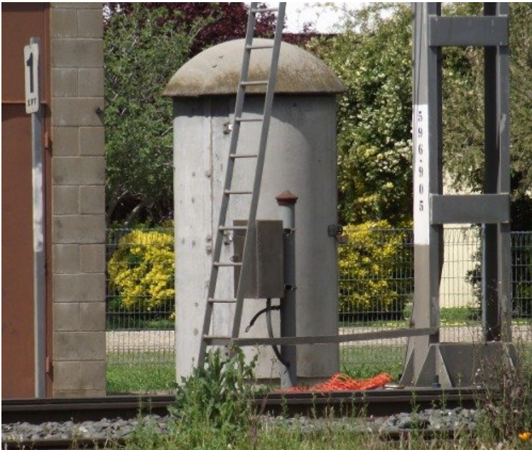
Above: Signalling circuitry shed (I think!)
